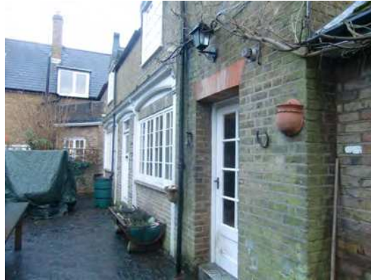
Picture 1.27 Original recessed doorway with gauged brick arch above - mirrored on the other side
